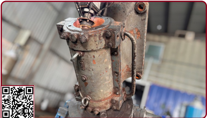
Bearing housing of the booster fan
